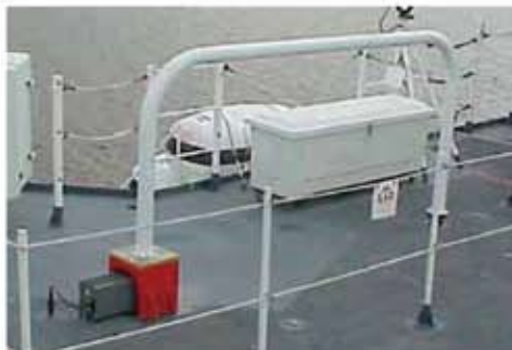
NVIS Antenna with TMR4096 Coupler
