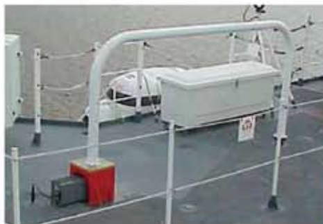
NVIS Antenna with TMR4096 Coupler
